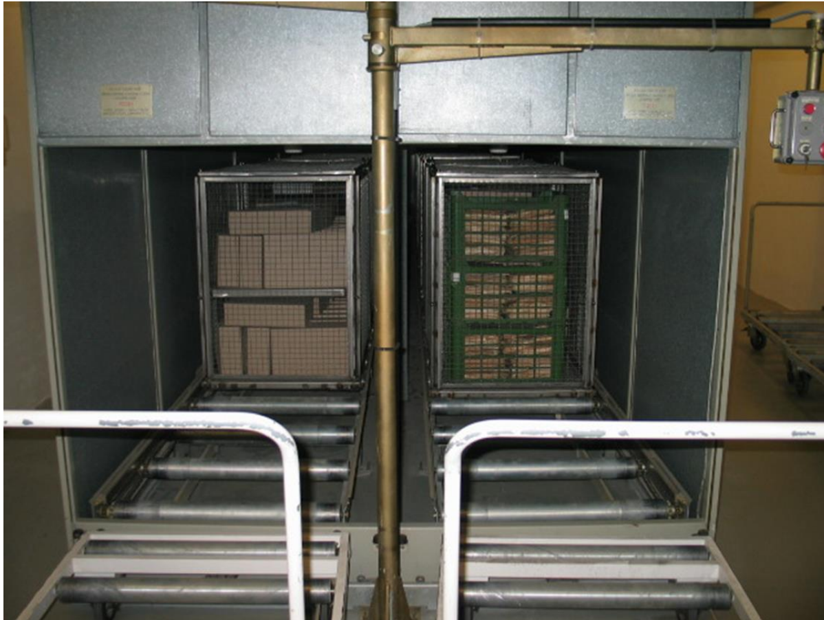
Tunnel for removing of ethyleneoxide
