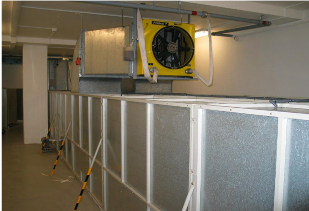
Tunnel for removing of ethyleneoxide
